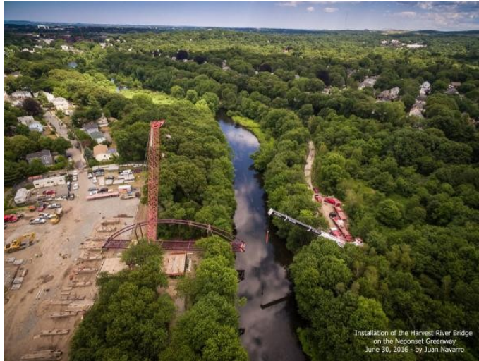
An aerial view of the Harvest River Bridge installation. Photo credit Juan Navarro
